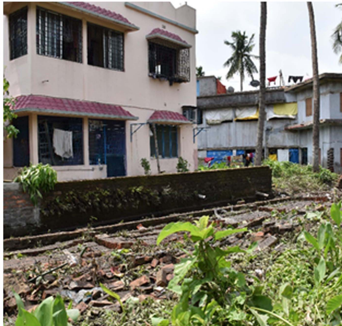
Oxford Mission-Sister side. East side of Sister House. About 120 Ft. length and 8 Ft. height boundary wall has collapsed.
